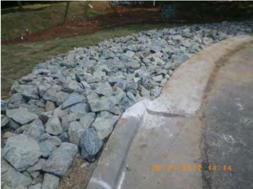
The driveway apron is cut flush and riprap laid at the entrance to the basin
